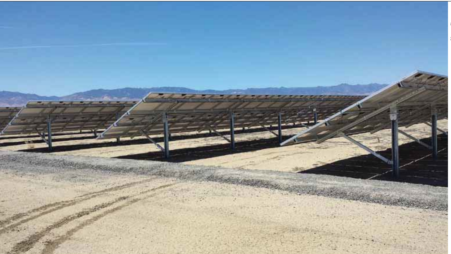
One way mounting system providers can gain attention for their brands is through advertising high-visibility installations, such as this project by Pacific Gas & Electric, which uses Clenergy's Terrace II mounting system.
